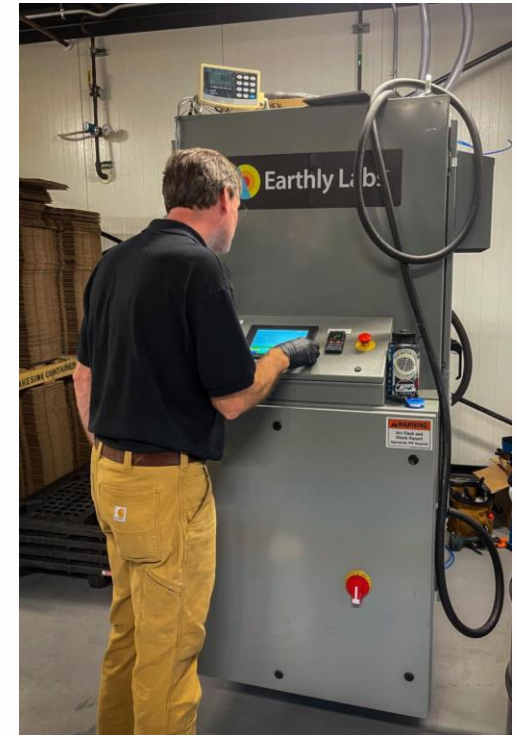
CiCi CO 2 Capture Unit Near Fermentation Tank Cellar
