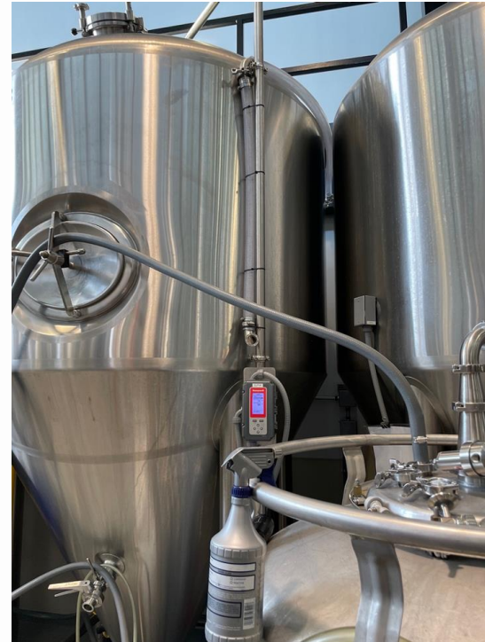
Blow-off Arm to Piping Grundy
