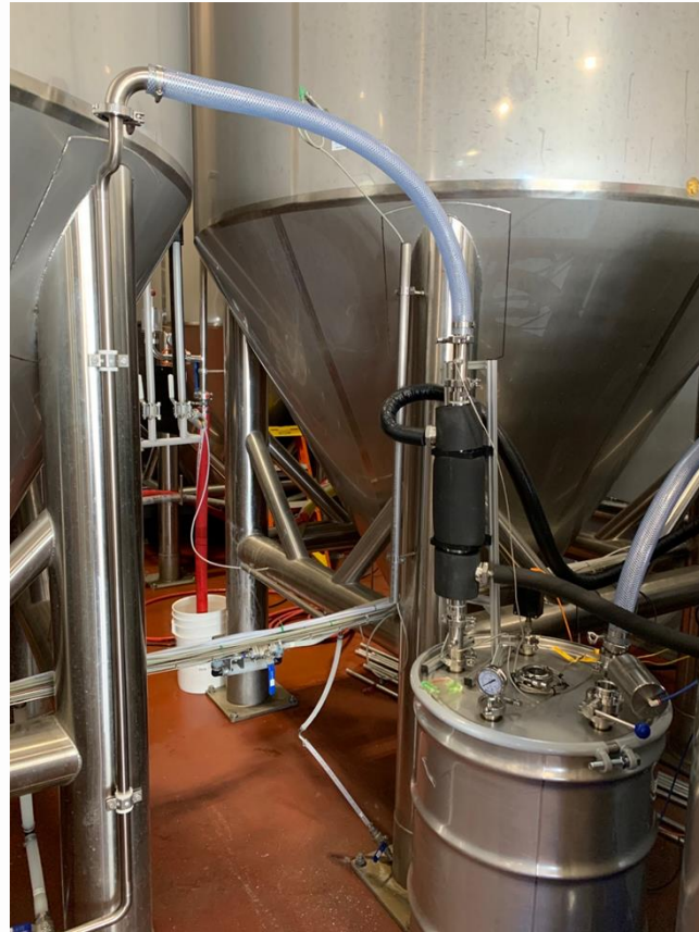
Foam Traps Capture CO2 at Fermentation Tank Blow-off Arm
